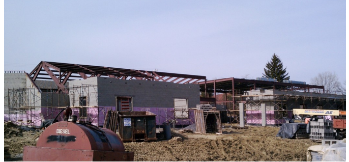
At right: The Salvation Army Community Center is on schedule for a June dedication. Photo provided by Laurette Underwood .
