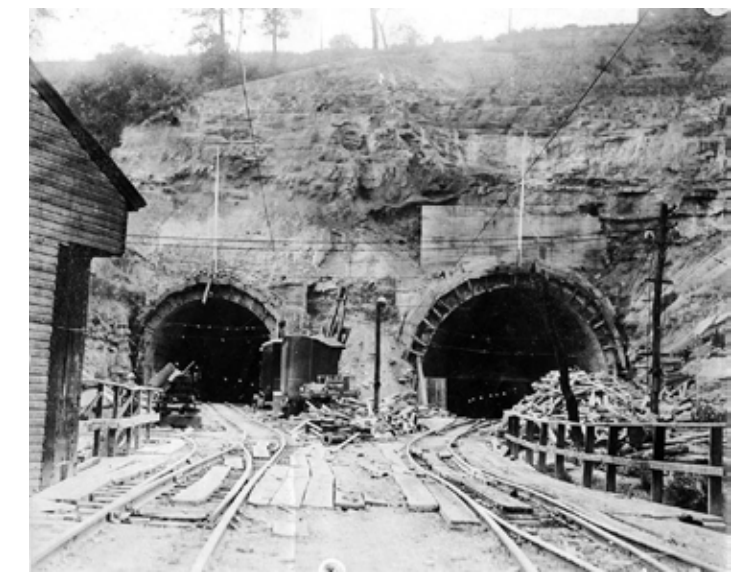
Boring proceeds on the Liberty Tunnels in 1922, as seen from the South Portal entrance along West Liberty Avenue. All images courtesy of The Brookline Connection.
